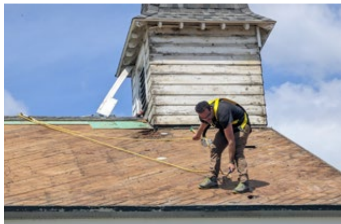
After removing all the shingles, a volunteer preps the roof for new roofing materials.
